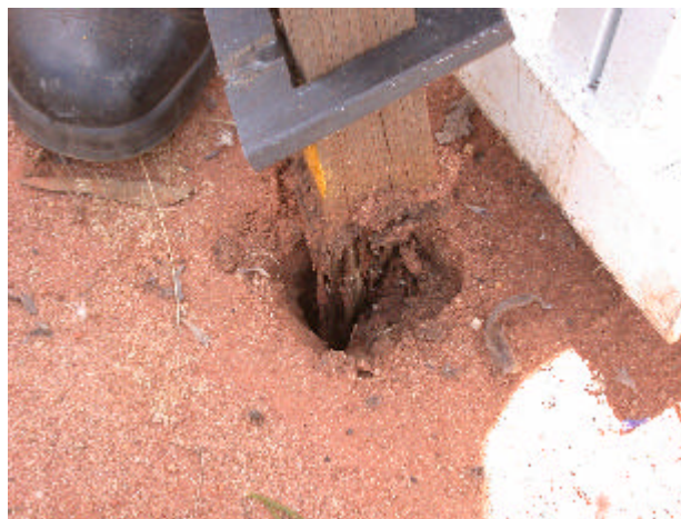
Figure 19. Specimen post with severe termite damage being removed at the Field Trial site.
