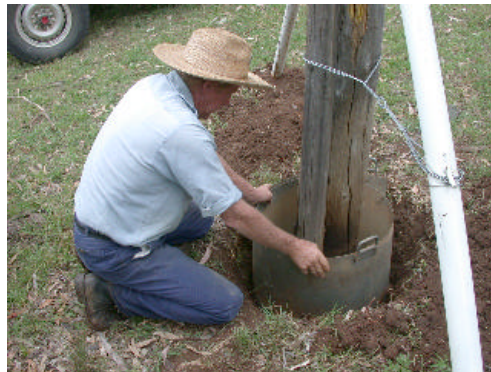
Figure 4. An adjustable cowling was used as formwork to maintain consistent barrier dimensions around each pole.
