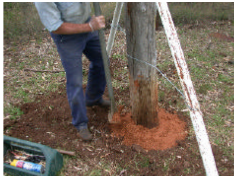
Figure 6. After the cowling was slipped out and removed from the pole, treated soil was compacted.
