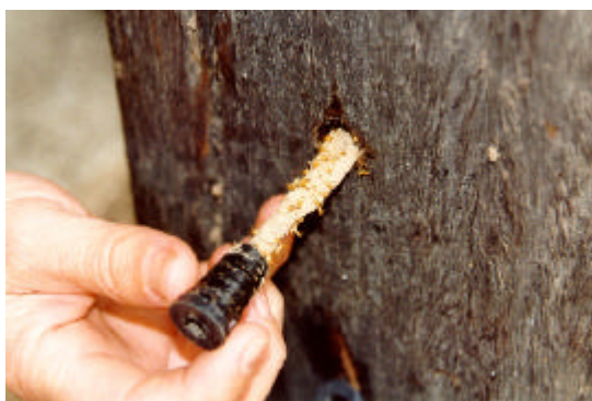
Figure 11. Baits made of radiata pine or mountain ash were used to detect termites in poles.
