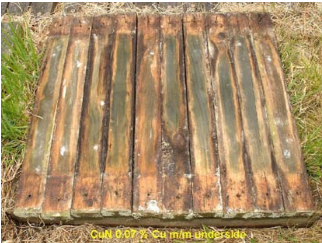
Figure 4. Copper naphthenate-treated P. radiata decking with 0.07% m/m copper after 13 years, underside.
