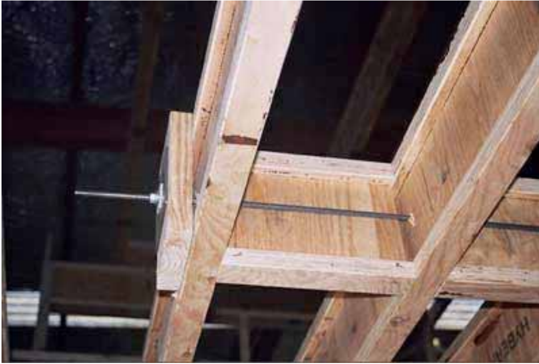
Floor 20. End of transverse beam before Hebel flooring in place, shows steel rod on central axis of beam
