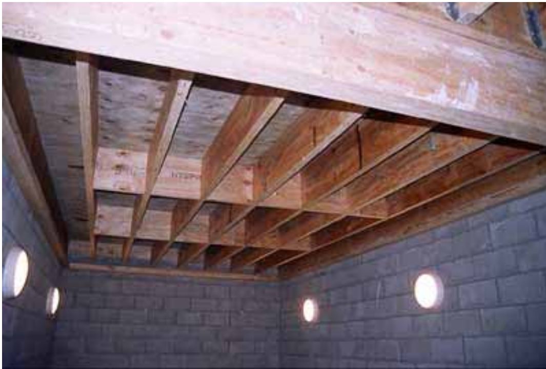
Floor 12. General view of underside of floor showing four transverse beams and cross beam supporting joists on both sides
