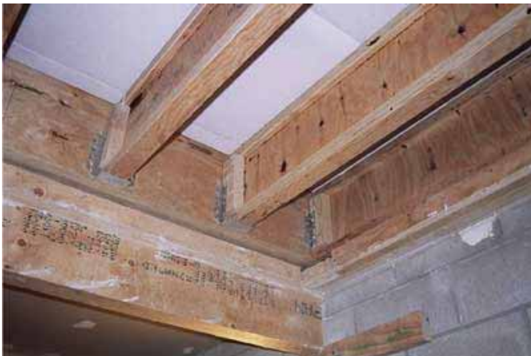
Floor 20. One end of joists supported on joist hangers off cross beam
