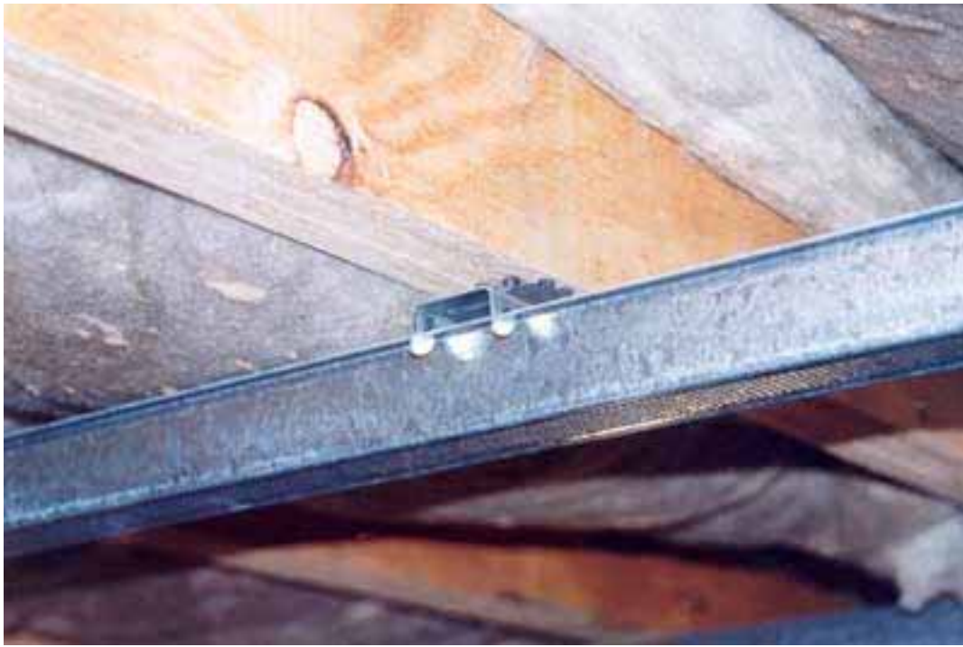
Floor 2. Close up of floor joist with RSIC clip to ceiling batten connection
