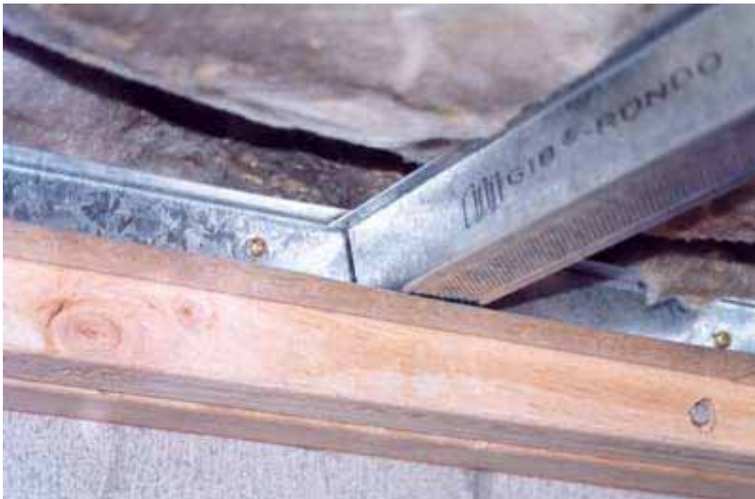
Floor 2. Junction of ceiling batten to steel J channel on to timber ground over blockwork
