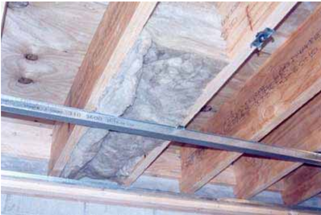
Floor 2. Ends of joists simply supported on timber ground with solid blocking. Also shown are steel batten, perimeter J channel, RSIC clips and fiberglass sound absorber in ceiling cavity
