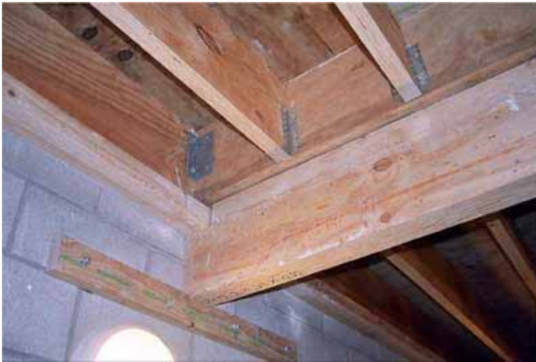
Floor 8. Cross beam above to support ends of floor joists with separate joist to support edge of ceiling
