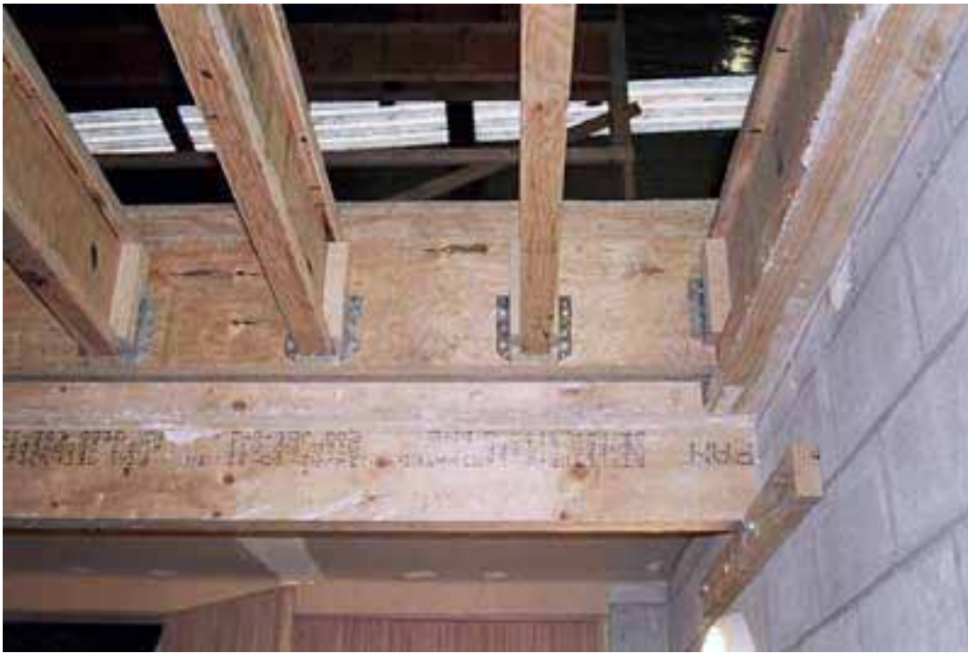
Floor 20. Ends of joist supported on joist hangers off the cross beam
