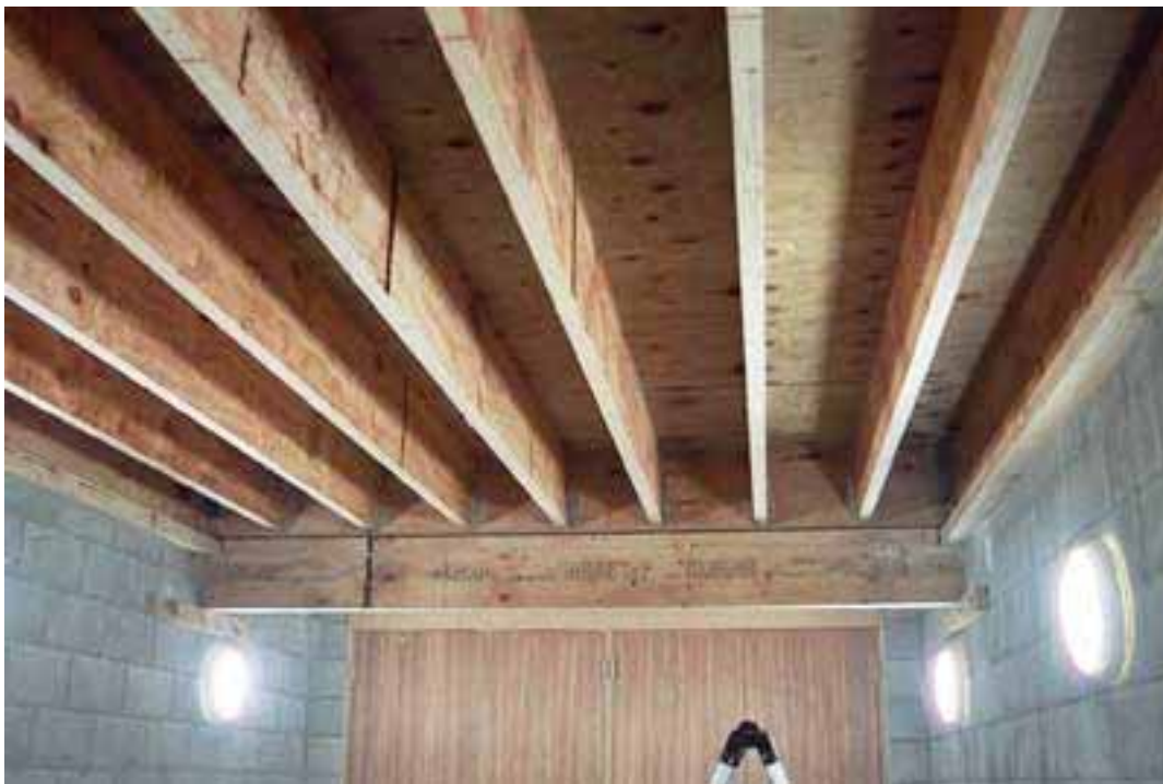
Floor 8. General arrangement of 300 LVL joists and support off cross beams with separate joist to support edge of ceiling
