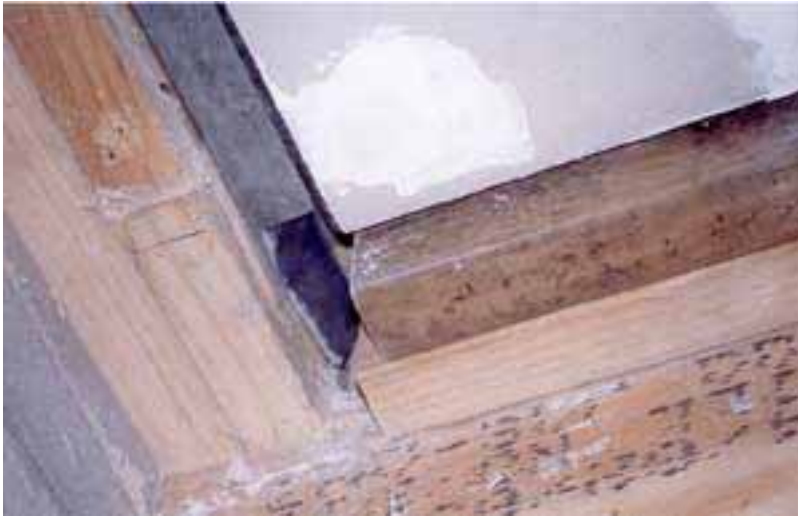
Floor 24. Close up of ceiling separation at corner
