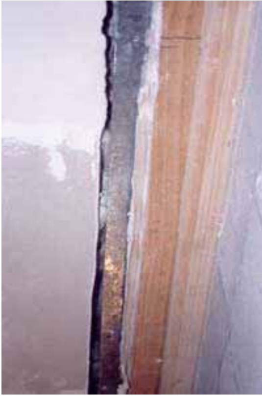
Floor 24. Ceiling separation at sides
