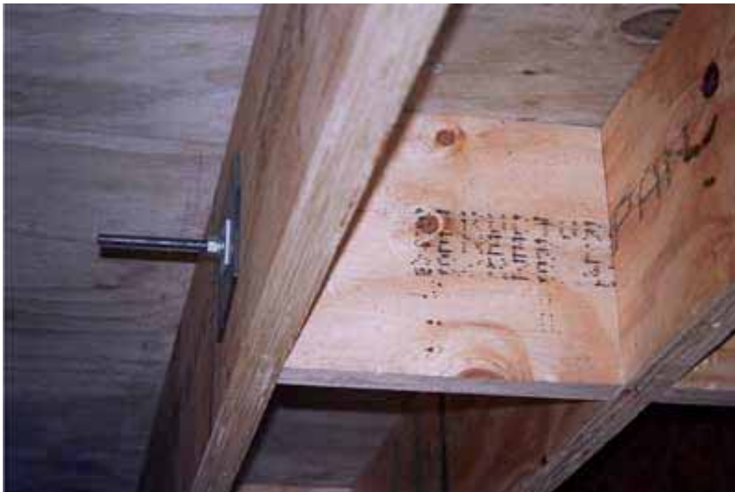
Floor 12. Shows solid blocking using 300x45 LVL and end of post tension rod on penultimate joist
