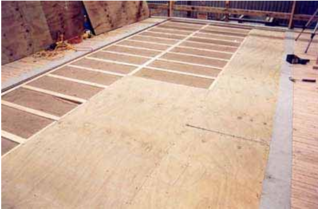
Floor 5. View of plywood flooring over 70x45 battens on flat with sand infill
