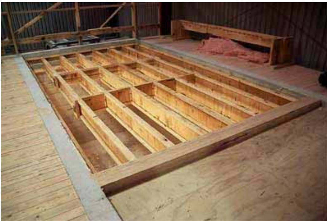
Floor 20. General view from above of 300 I joists with two transverse beams
