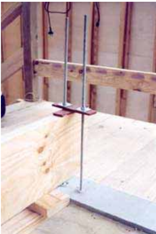
Floor 7. Close up of holding down bolts to end of clamping beam
