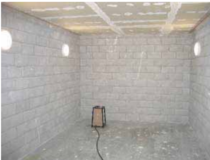
Figure 7-5. The scanning laser vibrometer as used to measure the vibration of the ceiling in response to the shaker force.
