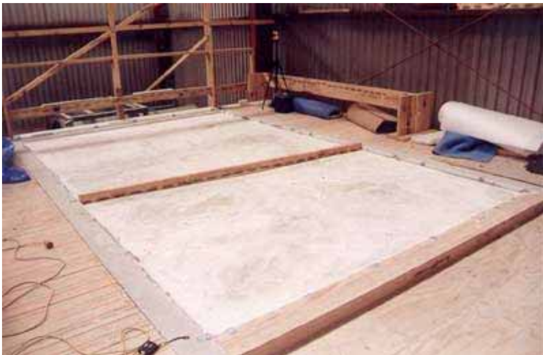
Floor 22. Completed gypsum concrete flooring, depth ranged from 10 to 46mm with average of 29mm thick
