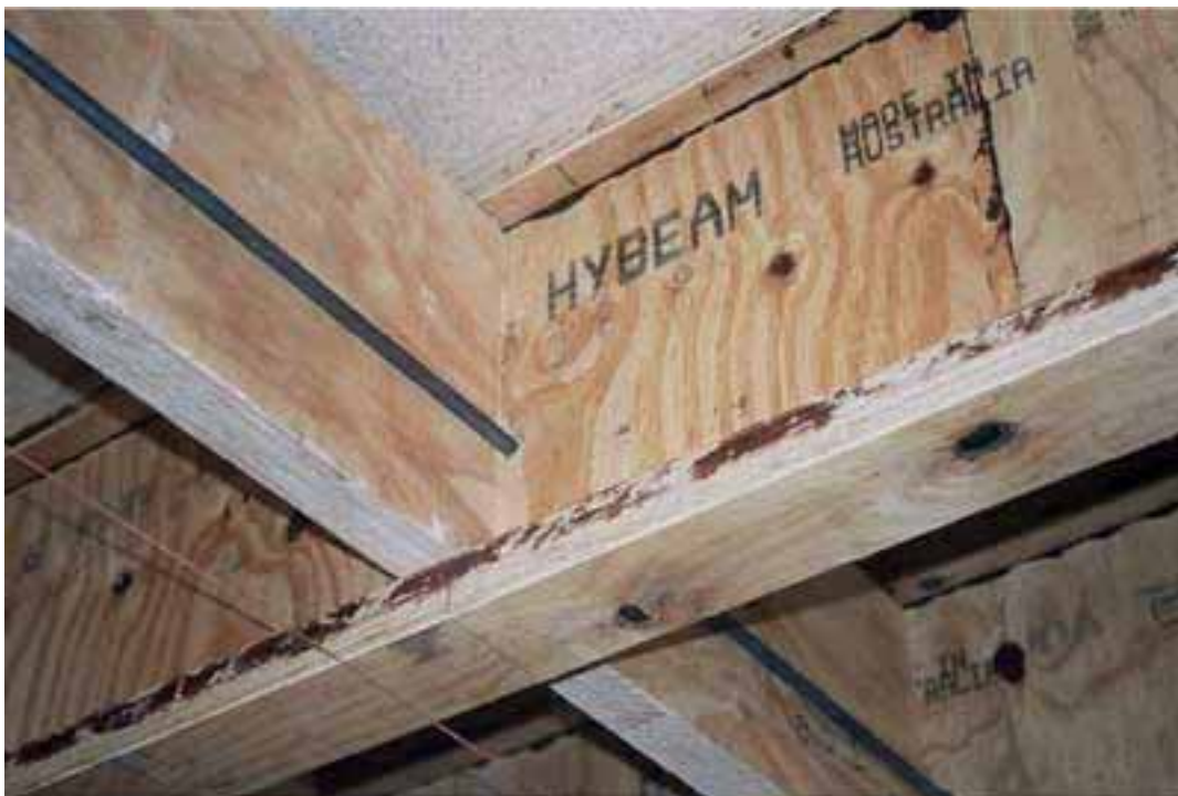
Floor 15. Floor joist to transverse beam junction shows steel rod below central axis of beam
