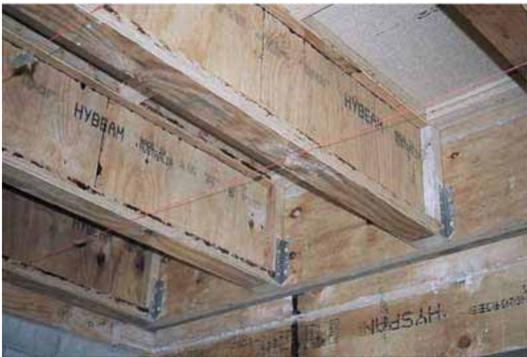
Floor 15. View of ends of 400 I joists supported on joist hangers off cross beam
