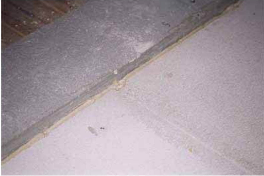
Floor 20. Junction of the Hebel floor to test rig reinforced concrete beam
