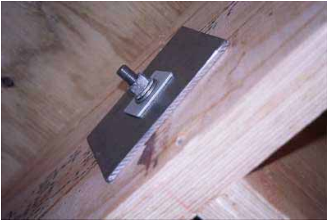
Floor 12. Close up of end of steel rod showing 150x150x10mm steel plate with 35x35 square washer, spring washer, washer and nut
