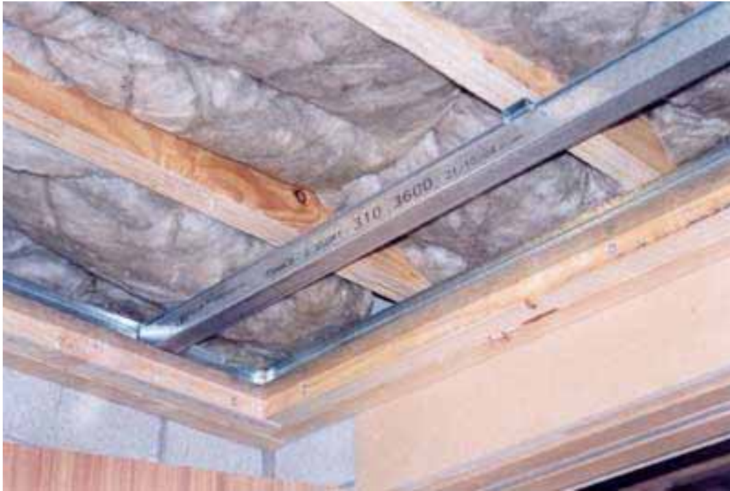
Floor 2. Shows steel batten spanning 800mm between RSIC clip and steel J channel
