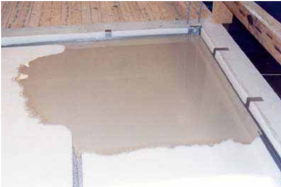
Floor 22. First pour of gypsum concrete on polyethylene foam underlay with taped joints
