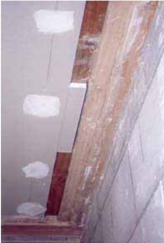
Floor 24. Ceiling separation at ends
