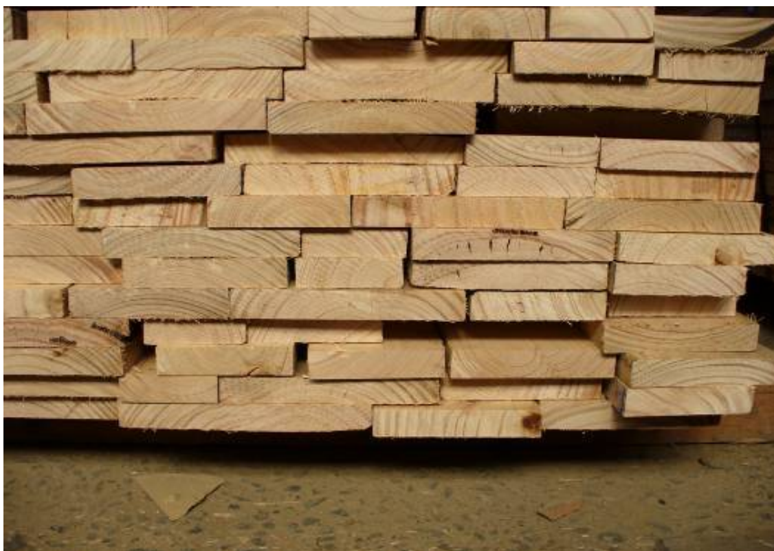
Figure 30. Internal checking in utility grade boards
