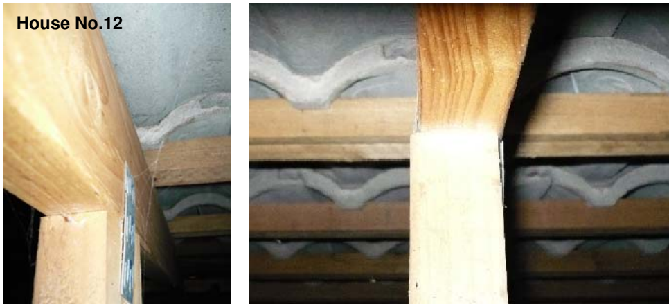
Figure 6.1 - A typical case of the 'alignment' type – the most common type found in the inspections
