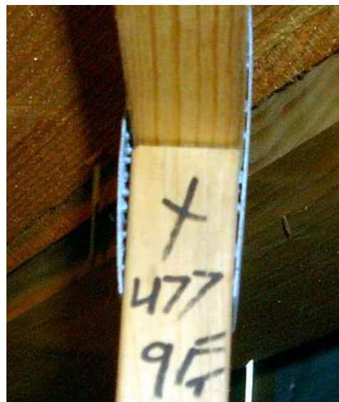
Figure 2.1 - Examples of nailplate backout inside roof spaces
