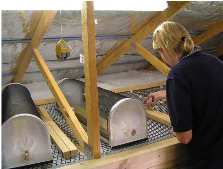
Figure 4: Cutting split-beams open for inspection in a roof space. A “Tiny Tag”™ datalogger can also be seen (Photo: L Vagg).
