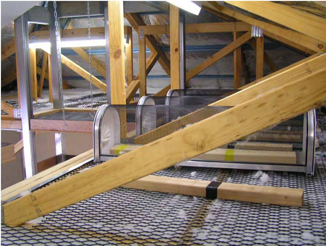
Figure 3: Roof space with cages and split-beams from trials 1 and 2 visible (Photo: L Vagg)
