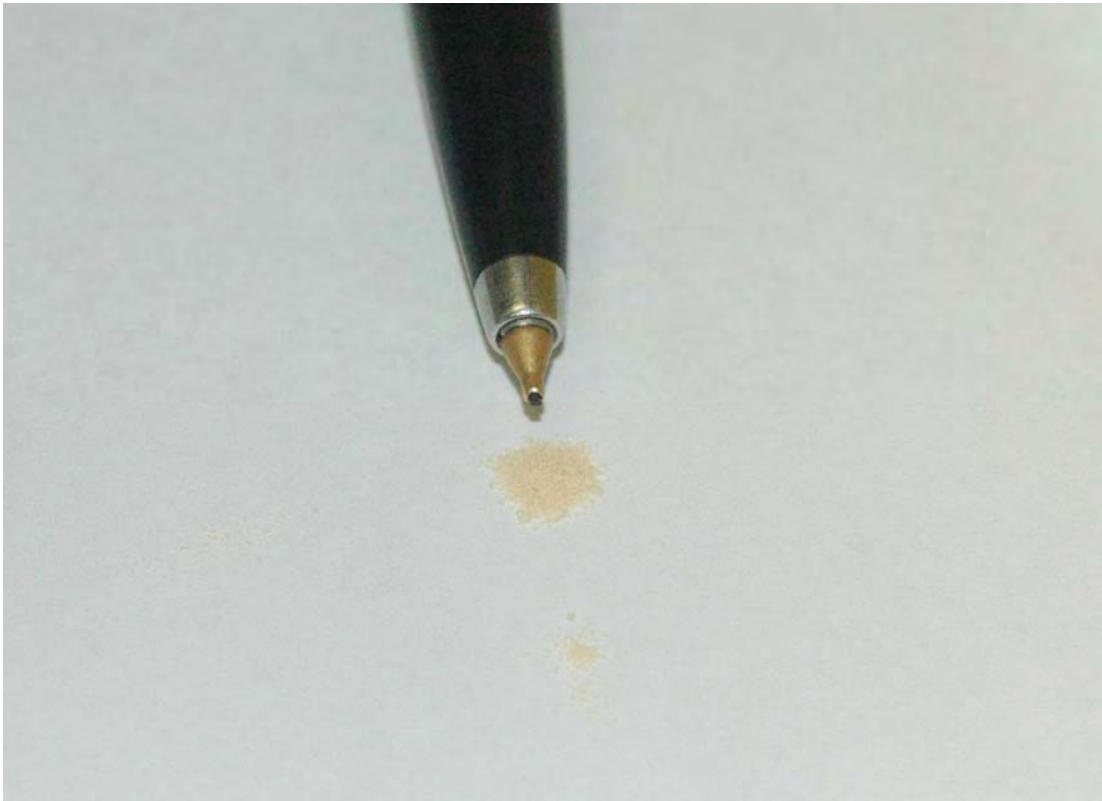
Figure 2: An excess frass pile found under a split-beam 18 months after initial infestation. This frass pile was produced by \approx 3 months feeding (April–July 2010). (Photo: RJ Cunningham)
