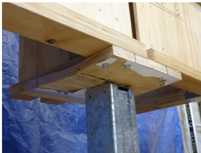
Figure 12. Plywood plate ruptured
