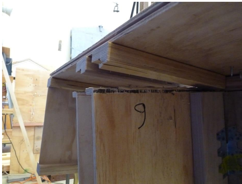
Figure 14. Joist web pulling out of flange
