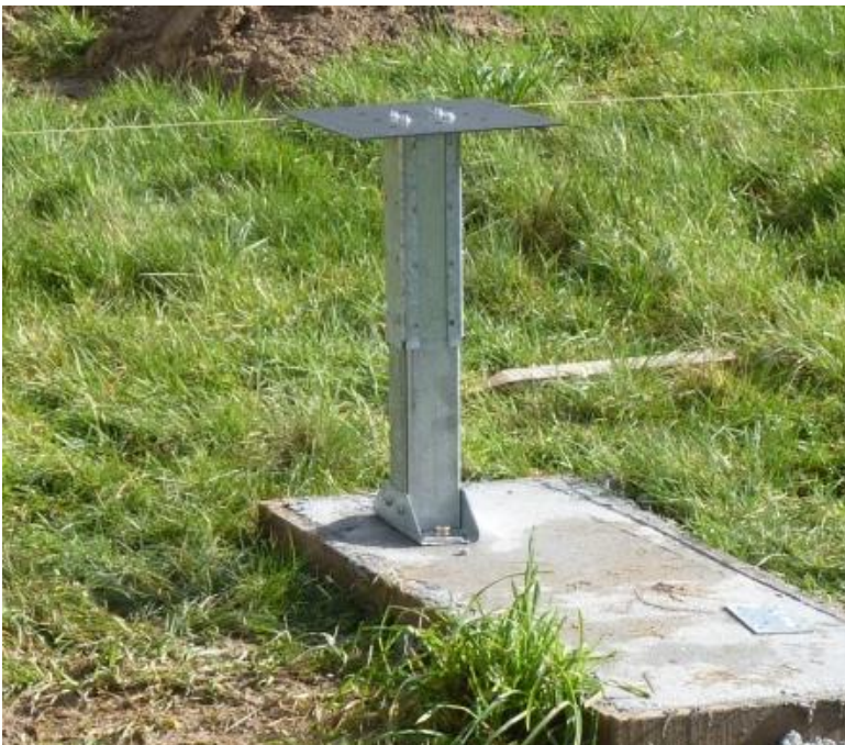
Photograph 4. Steel support pier. Note upper telescoping section screwed to connector plate
