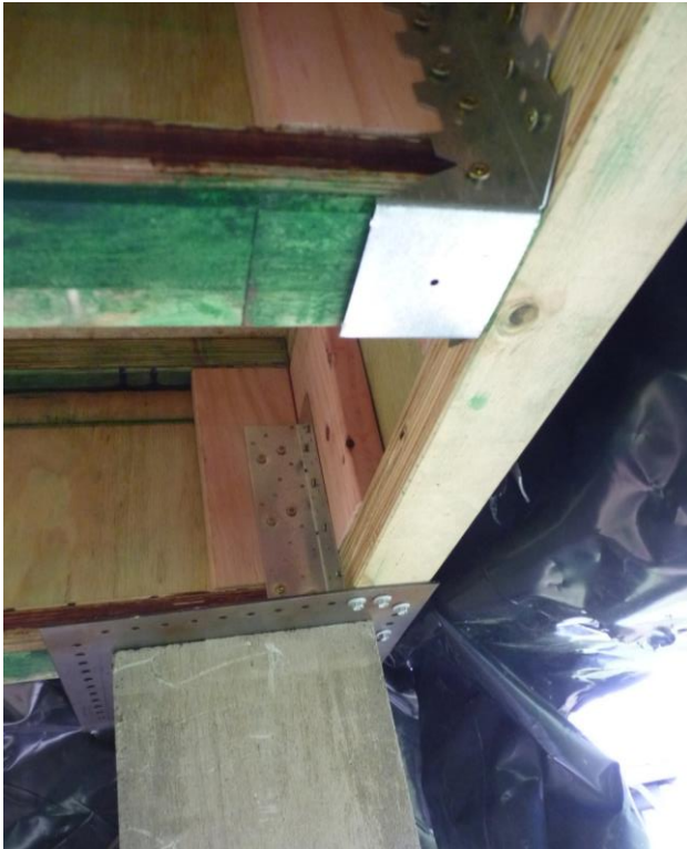
Photograph 2. Connection detail beneath floor panel. Note joist hangers, nailplate connection between boundary joists, and screw connection to concrete support and plate.
