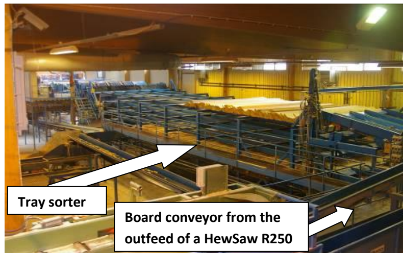
Figure 23: A tray sorter installed at the Havesa Timber sawmill, Hamina, Finland. The sorter can pick up boards and transports them sideways from the conveyor at the end of a HewSaw R250 without elevation of the boards. The tray sorter is an alternative to sling sorters that may cause problems for handling bowed eucalypt boards (source: Washusen 2008).
