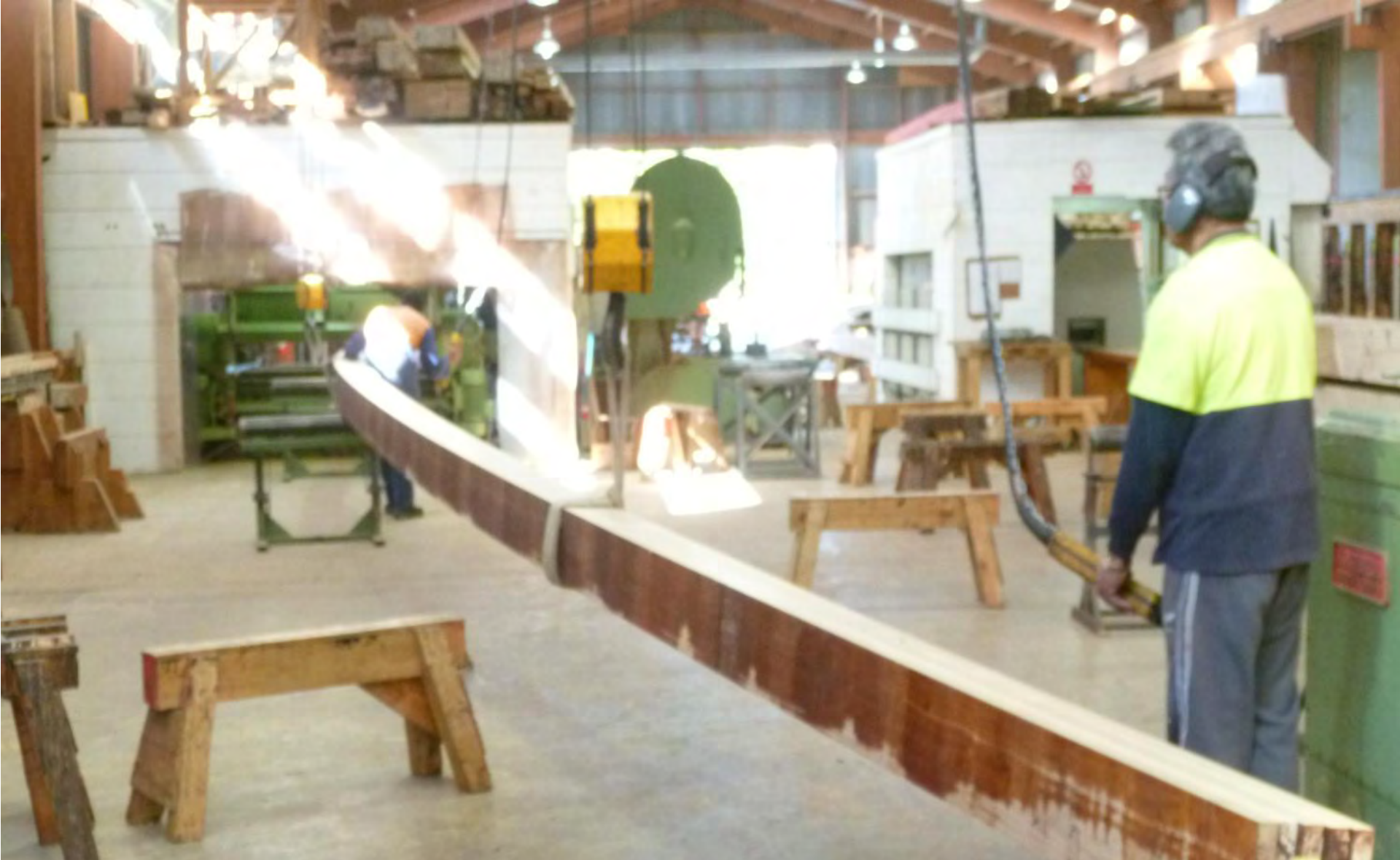
29m beams – curved and twisted
