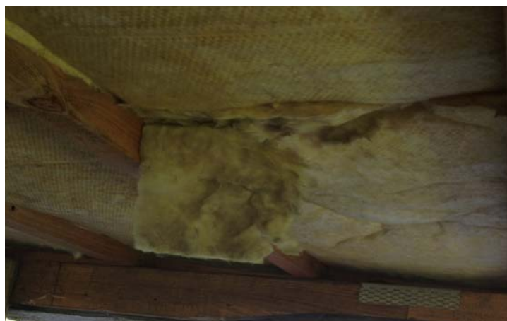
Figure 14: Delamination of glass-wool subfloor insulation batt
