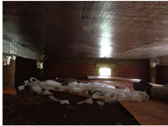
Figure 2: Manufacturer installed reflective subfloor insulation
