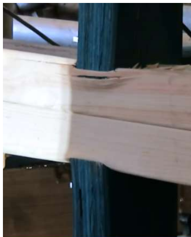
Figure 24: Large deformation of MGP10 Wall Plates
