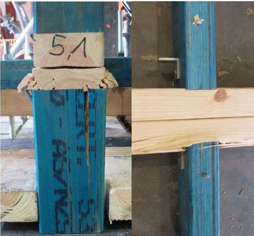
Figure 36: Splitting of the LVL stud by the screw reinforcement
