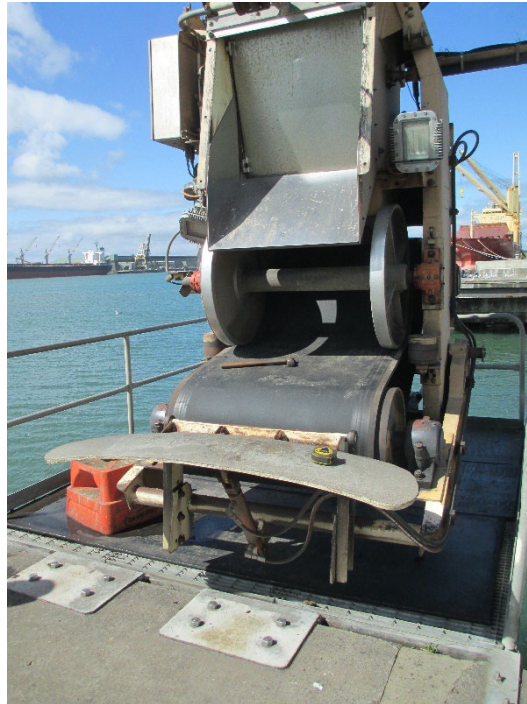
Jet slingers distributing chips to a woodchip pile (top) and undergoing repairs to a deflector plate (bottom).
