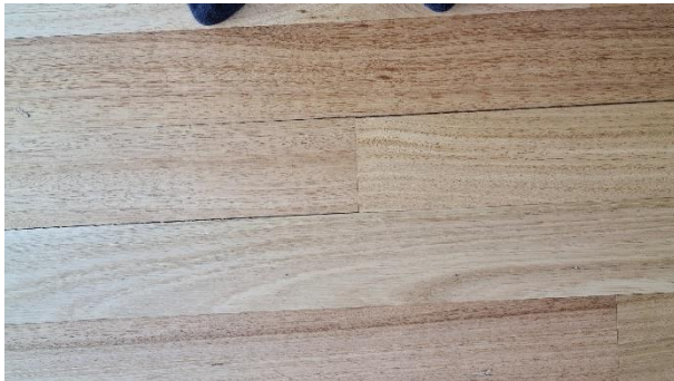
Figure 3: Minor slabbing from board adhesion.
