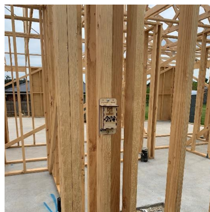
Figure 15: Sensor-only unit on a timber frame.
