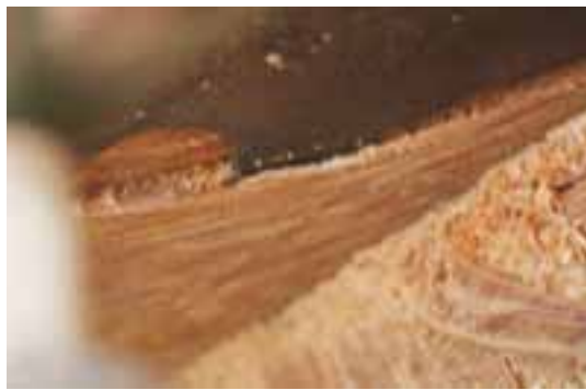
Fig. 5.18: Tooth in timber showing removal of sawdust.
