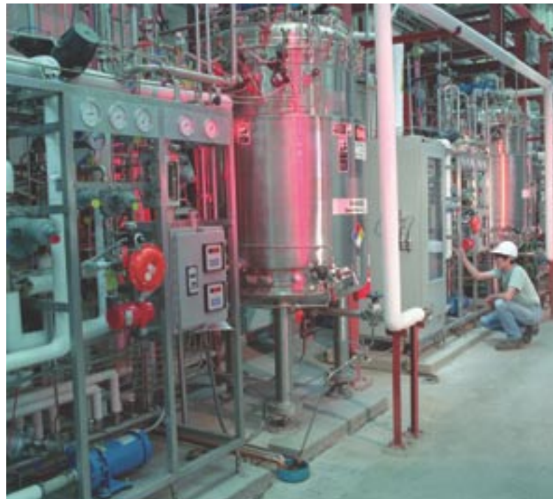
Wood to ethanol pilot plant
